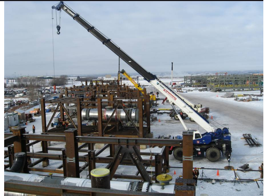
77 acre fabrication yard in Sherwood Park, Alberta
